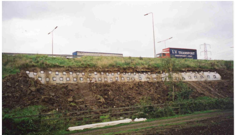
Duckbills installed in an embankment on the M25 near Junction 29, the A127 in Essex
