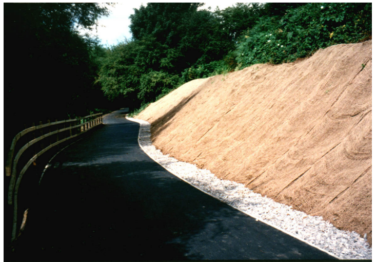
The completed cycle route with geogrids and top soil in place on the fully stabilised embankment.
