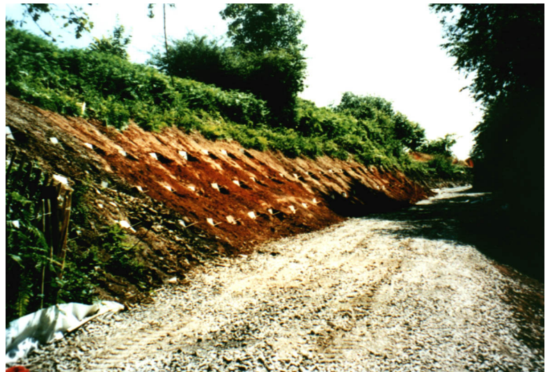
The load plates remain visible on three rows of Duckbill MR2 stainless steel anchors following installation to secure the embankment.
